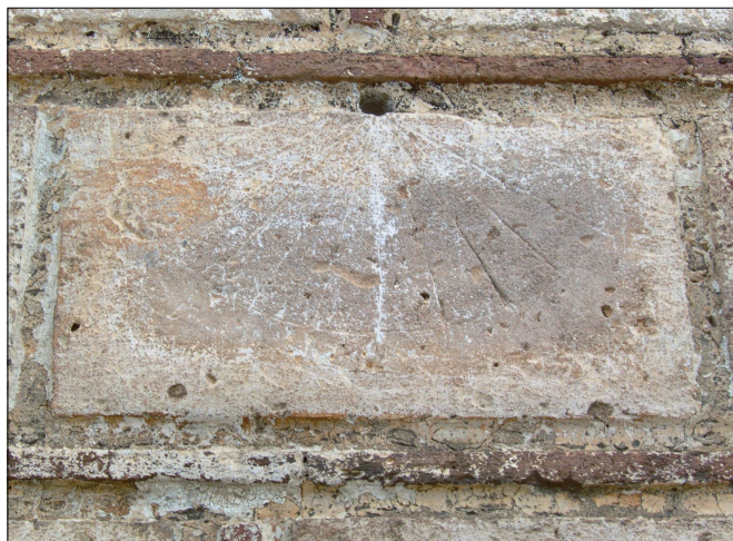
Fig. 3. The weathered mass dial at the Chonikas church. It is on the 7 th stone counting from the double base of the building and the 3 rd from the SE corner.
